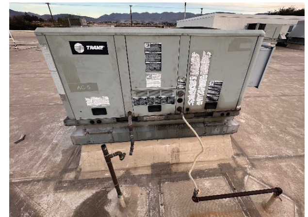
PHOTO: Packaged A/C Unit
