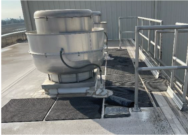
PHOTO: Mechanical Roof Unit
