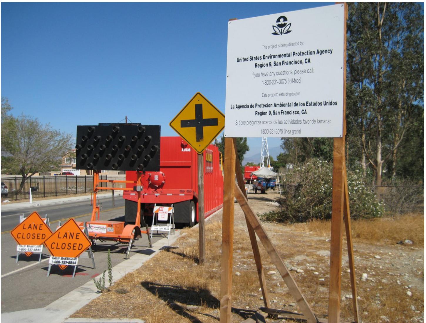
Groundwater Monitoring Well Site in Rialto, CA.
