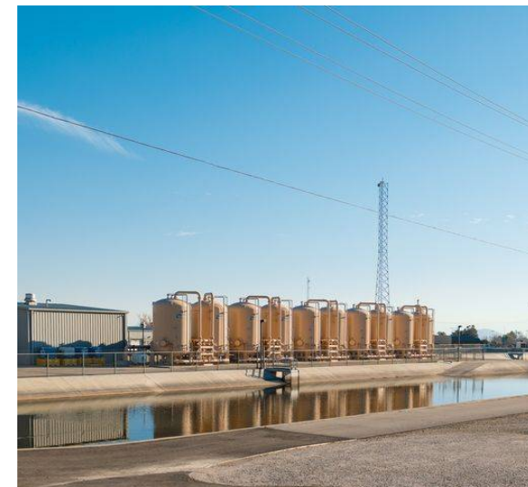
Roemer Treatment Plant
